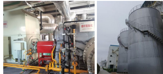
On-Site Screw Expander and Hot Water Storage Tanks
