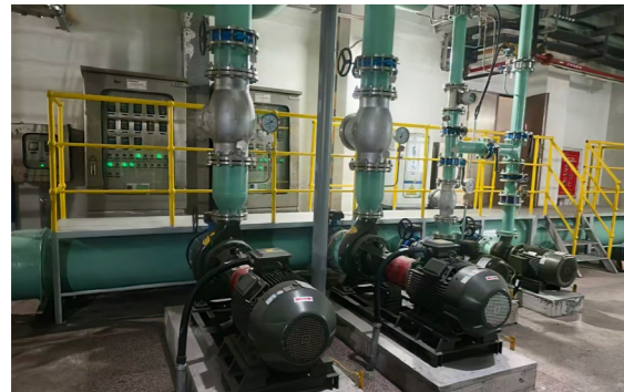
On-Site Secondary Reverse Osmosis Feed Water Pumps and Flush Pumps
