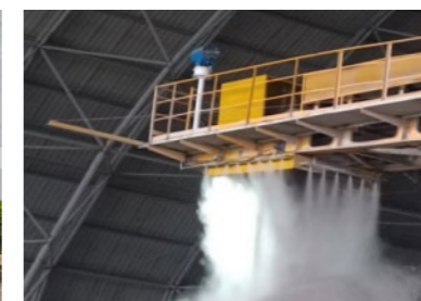
Application of Dry Fog Dust Suppression at Stockyard Feed Point
