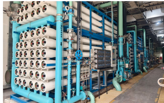
On-Site Secondary Reverse Osmosis Units
