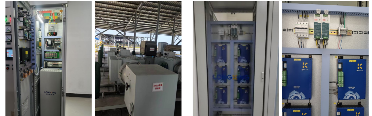
Electrostatic Precipitator Variable-Frequency Power Cabinet
