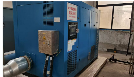
Oxidation Fans of the Desulfurization System
